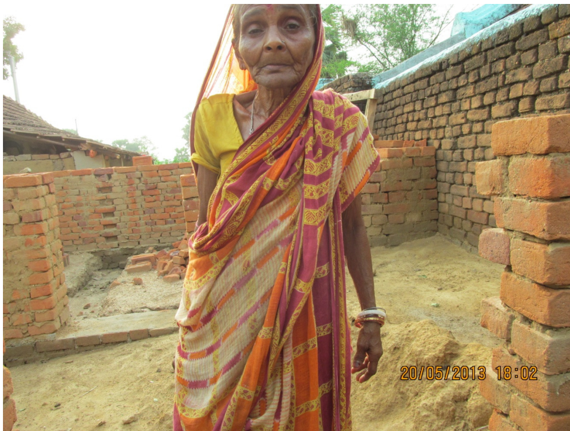
Under Construction IAY House of Mrs. Dipali Bauri, Village-Siju Makhana, Keshargarh Block-Hura, Purulia
